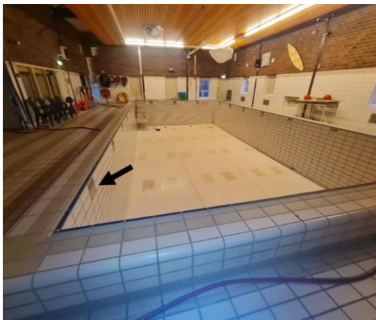
Lekkage in skimmer (foto Triton)
