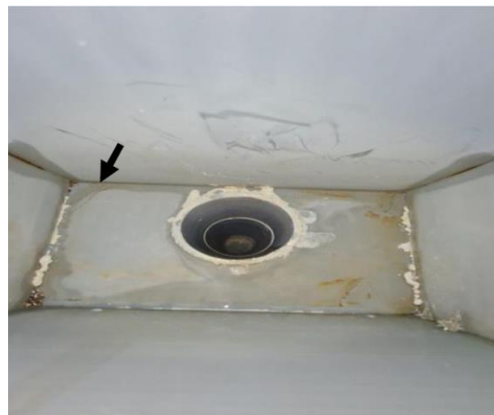
Lekkage in skimmer (foto Triton)
